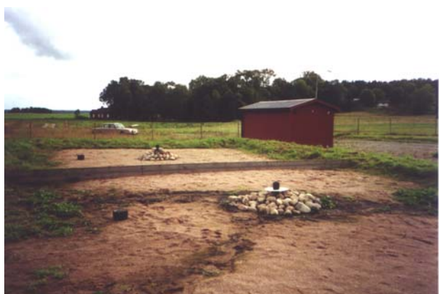
Box 4.3: An open sand filter in Lagga
