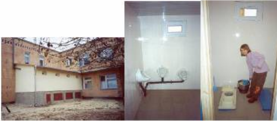
Figure 4.9. New school toilet in Gozhuly village: outside (left), urinals (centre) and inside (right).
