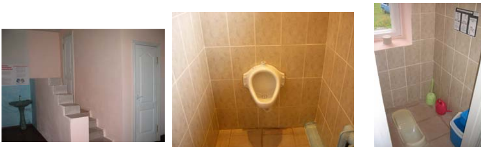
Figure 4.11. New school toilet in Bobryk village: outside (left), urinals (centre) and inside (right).
