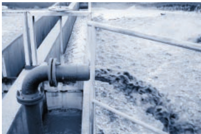
Sewage treatment plant, Podgorica, Serbia and Montenegro
